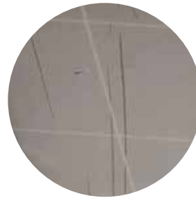
Outer-layer cracks 7 years, SW USA
