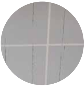
Outer-layer cracks 6 years, NW China
